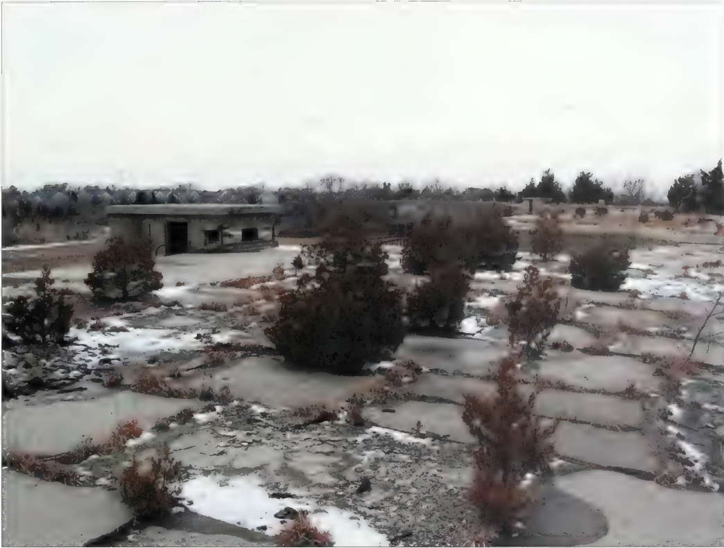
Figure 3.21. View looking west toward battery commander's station Bloomfield, Nine Gun Battery. In addition to growing on the engineered earthwork, eastern red cedars ( Juniperus virginiana ) have emerged in the cracks and cold joints of the battery's horizontal concrete surfaces (Olmsted Center, January 2009).
